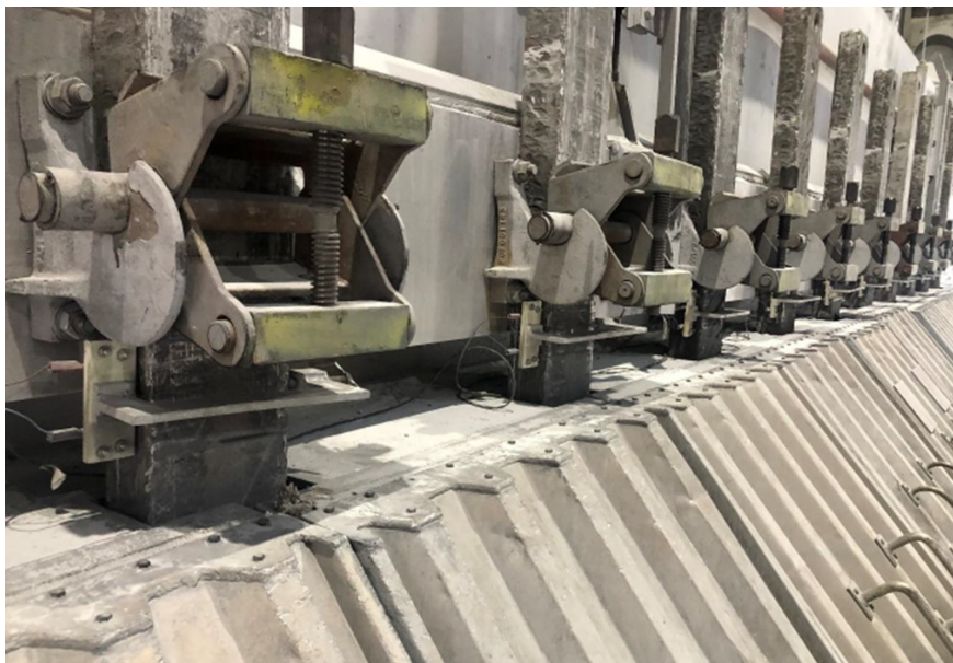
Figure 5. C-clamps installed on the anode rods of cell upstream side.
