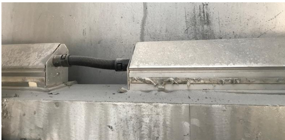
Figure 2. Sensors on the anode beam are enclosed in a channel for additional protection against dust particulates and moisture.
